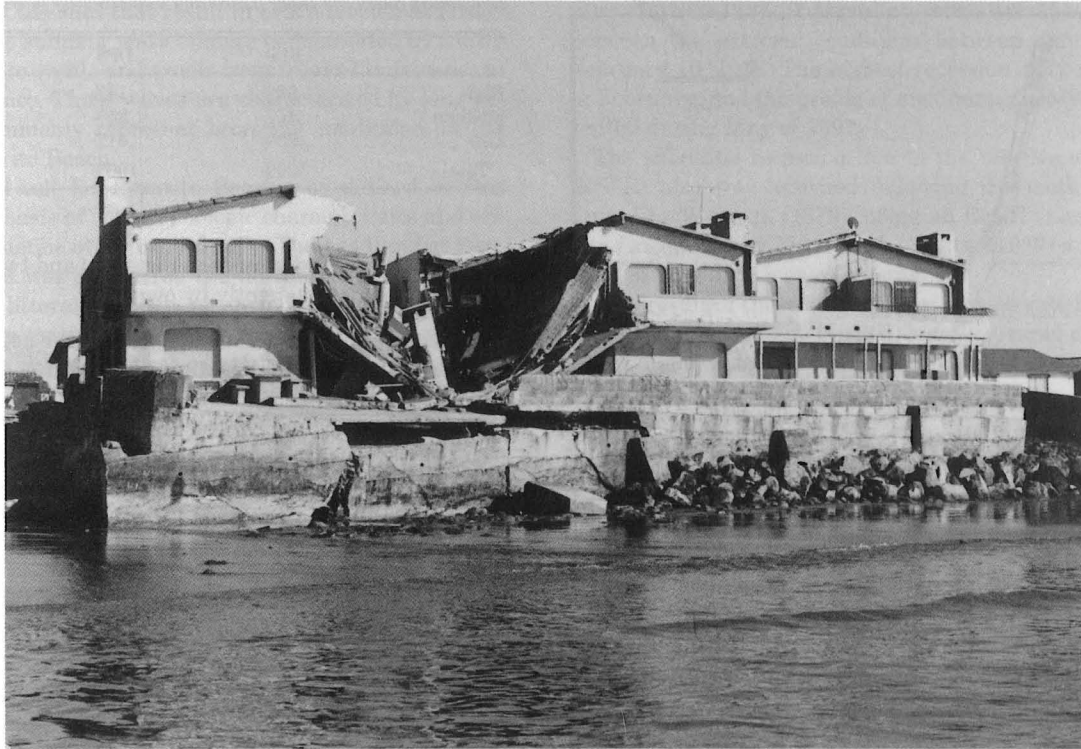
Figure 3. Localized damage in a high vulnerability area, February, 1998.
