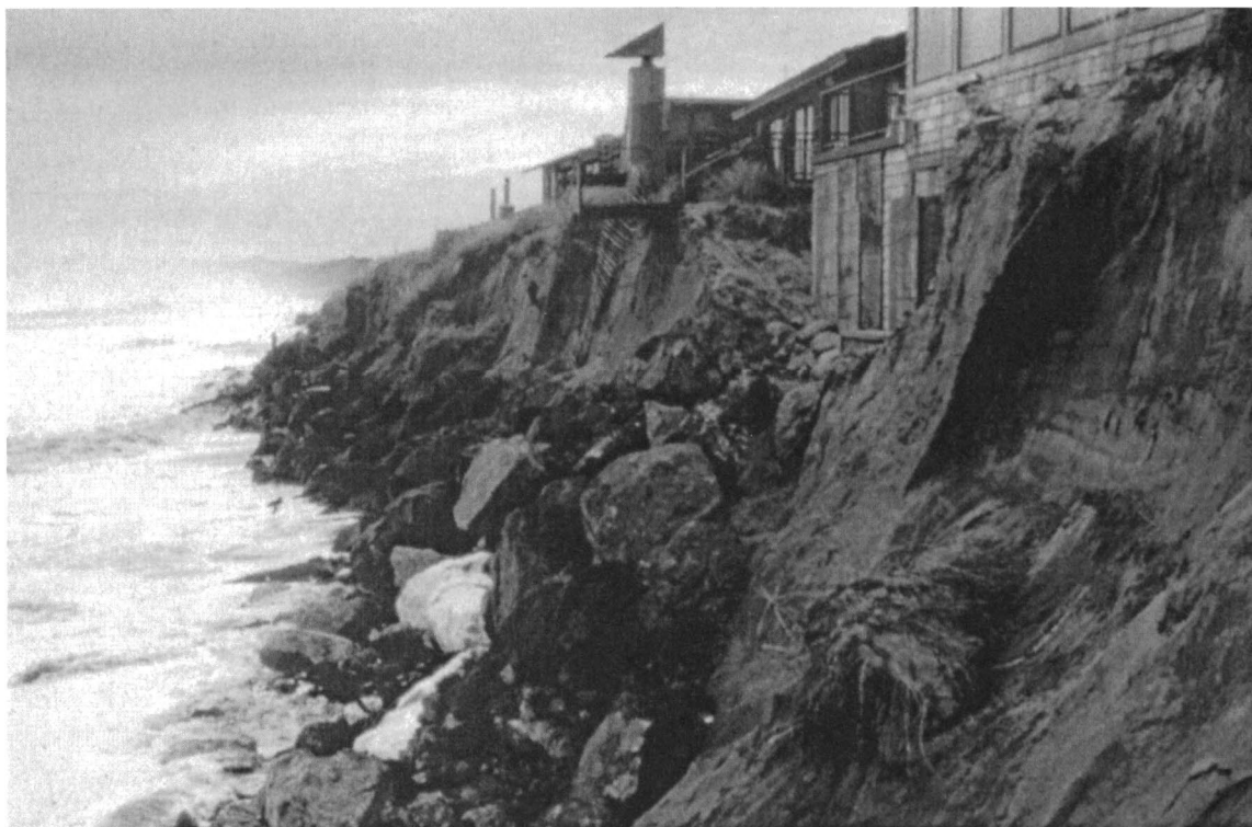
Figure 3. Beach and dune erosion at the Pajaro Dunes development in early 1983. Over 15 m of the dunes were eroded during the storms of early 1983, undermining the foundations of many structures. The rip-rap was emplaced at the height of the storms to stop further erosion and the possible collapse of structures.
