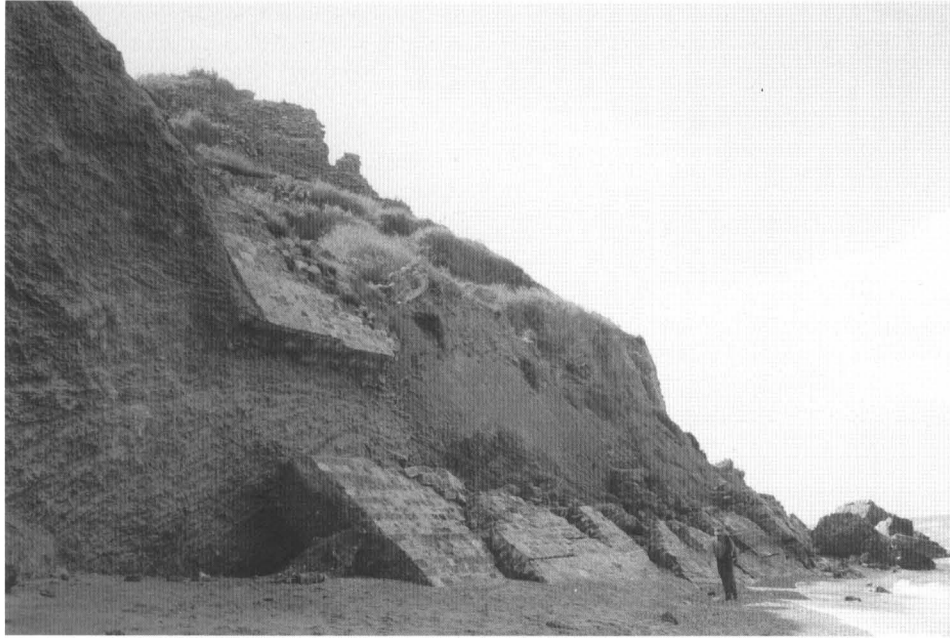
Figure 6. Slabs of cemented masonry lining the defensive moat of the 13th century castle of Arsuf. The detached slabs slumped onto the beach in late winter 1994.
