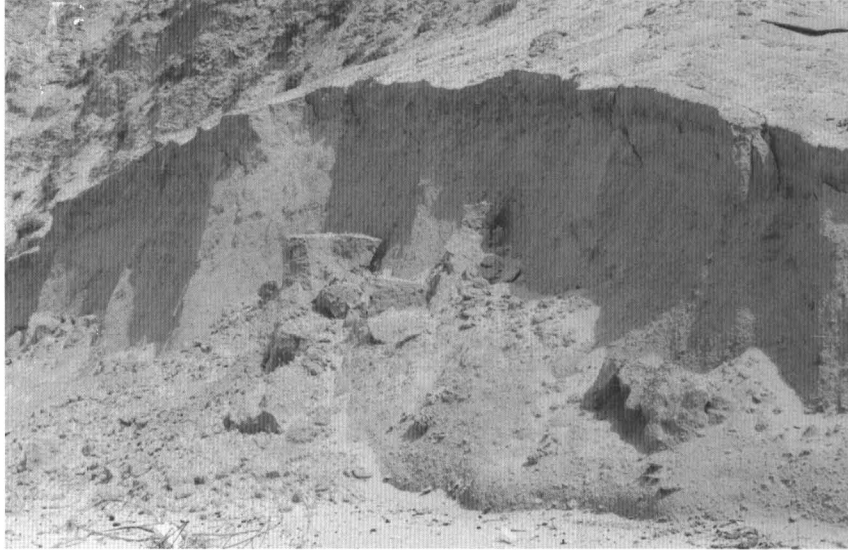
Figure 10. Wave-cut step, truncating the toe of a sandy talus apron (Risk B). The step is maintained at this high angle by capillary forces in the moist sand. Desiccation results in collapse, as has happened to the apron in the foreground.
