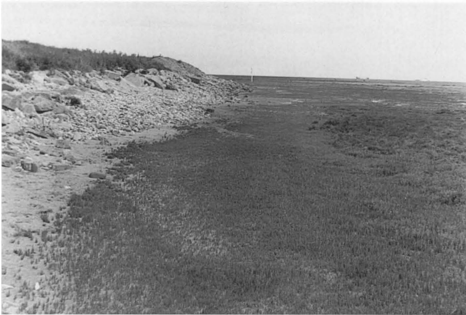
Figure 11. Erosion damage to the 1979–1980 embankment at Frinskney where the fronting saltmarsh between two former creeks is slightly lower than on either side. Photograph taken in July 1992.
