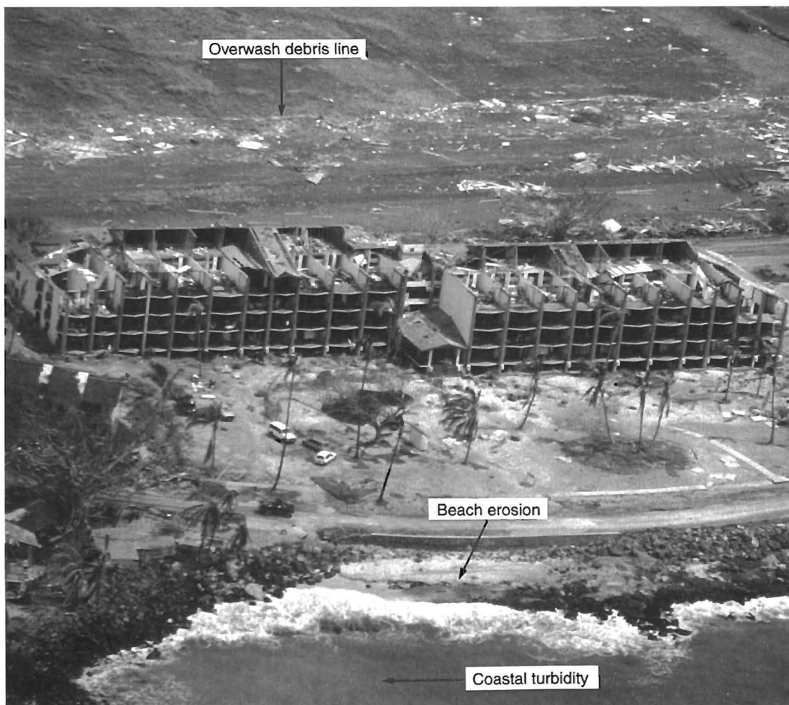
Figure 1. An 80 unit condominium complex, lower floors destroyed by overwash, upper floors destroyed by wind. Note the overwash debris line in the background. East of Kukuiula Bay, Kaua'i.
