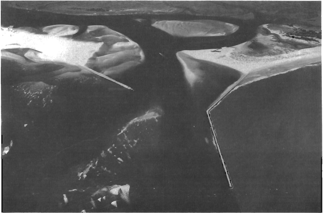
Figure 8. Aerial photography showing channel configuration during construction of the west jetty: September 1982.
