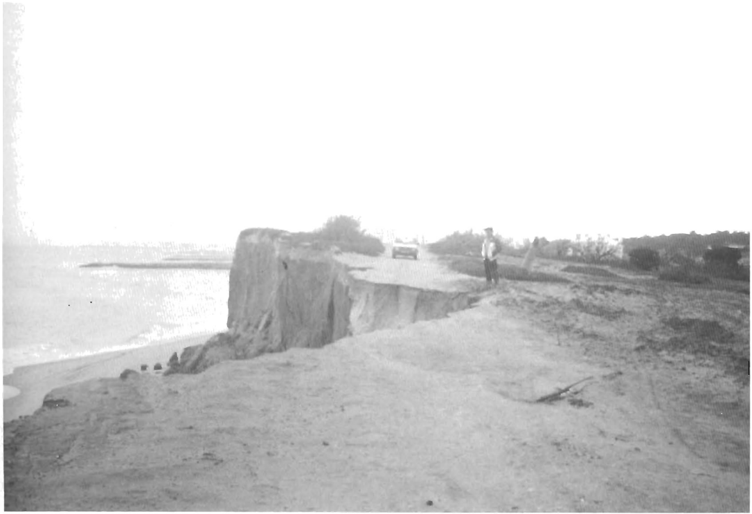
Figure 5. Missing section of road along the cliff edge due to rock fall/slump.
