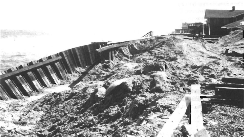
PHOTO 182. Collapse of the Sandbridge, Virginia, bulkhead. Upper photo: Newly constructed steel sheet-pile bulkhead on 25 January 1989 at Sandbridge, Virginia. The bulkhead is constructed of 7.6-m long steel sheets which stand above 4 m. The base of the wall extends into a salt marsh peat layer. The wall has 5.5-m tie-backs, but no filter cloth. Lower photo: The same Sandbridge bulkhead on 10 March 1989. Failure is attributed, in part, to the peat substrate. (Photos: David Kaiser and Kathie Dixon, Department of Geology, Duke University, Durham, NC 27706).
