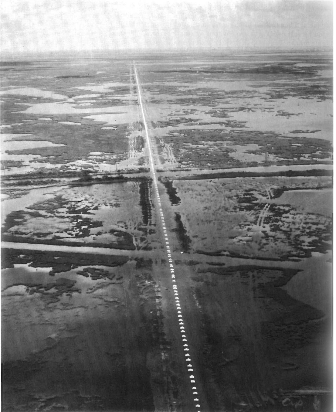
PHOTO 111. The LOOP (Louisiana Offshore Oil Port) pipeline being laid across the coastal marshes of Louisiana. (Photo: Don Davis, Department of Geography & Anthropology, Louisiana State University, Baton Rouge, LA 70803).
