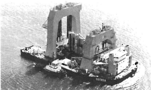
Figure 25. A specially designed vessel, Ostrea , transports a gate-support pier from the flooded cofferdam construction yard on Neeltje Jans, to the Eastern Scheldt barrier alignment. (Photograph by Bart Hoffmeester, Aerocamera. Rijkswaterstaat Meetkundige Dienst Afdeling Reprografie).
