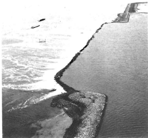
Figure 23a. A critical section of Marquisate Quay under construction on the Scheldt-Rhine waterway link. Note the strong tidal flow through placed-fill core materials in the closure dike. (After Rijkswaterstaat, 1987).
