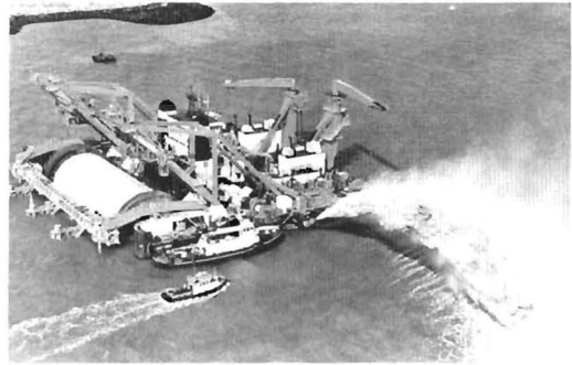
Figure 28. As part of the foundation for the Eastern Scheldt barrier, a specially-designed barge was used to lay down filter mattresses on the prepared seabed (from reel on the aft-end of the barge). Drawing shows: (1) foundation mattress being unrolled, (2) weighted beam which holds the end of the mattress in place, (3) small surface compactor and (4) a small leveling dust-pan dredge. (Photograph by Bart Hofmeester, Aerocamera. Rijkswaterstaat, Meetkundige Dienst Afdeling Reprografie).
