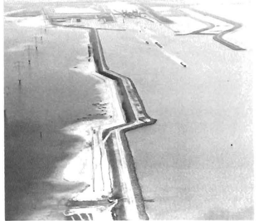
Figure 23b. A dredged-sand embankment over the rubble core completes the dike and eliminates a tidal influence on this section of the waterway. The Kreekrak lock system is in
