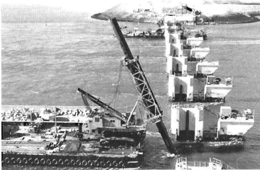
Figure 32. Larger armorstone rip rap had to be placed by a special vessel to avoid damage to piers. (Photograph by Bart Hofmeester, Aerocamera, Rijkswaterstaat Meetkundige Dienst Afdeling Reprografie).
