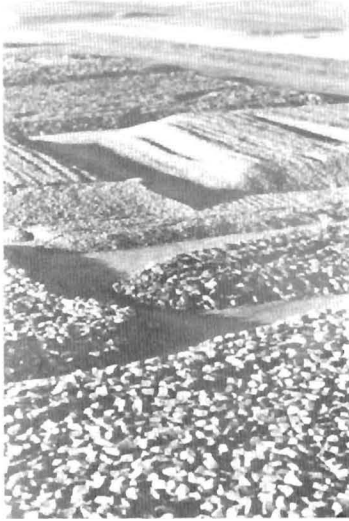
Figure 31. Some five million tons of rock rip rap were imported from quarries in Belgium, Finland, Germany, and Sweden to protect the foundations and lower sections of structural components of the Eastern Scheldt barrier. (Rijkswaterstaat Meetkundige Dienst Afdeling Reprografie).
