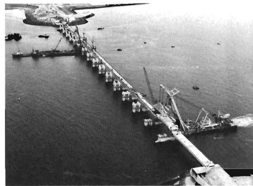
Figure 33 cont. (b) Installation of a road-section box girder (Photograph shows the barrier across one of the three channel sections of the Eastern Scheldt estuary).
