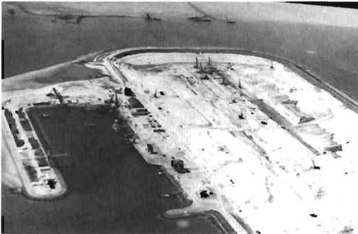
Figure 21a. Haringvliet cofferdam and dewatering system enabled piled foundations and sluice-gate support piers to be constructed in the dry. (Rijkswaterstaat Meetkundige Dienst Afdeling Reprografie).
