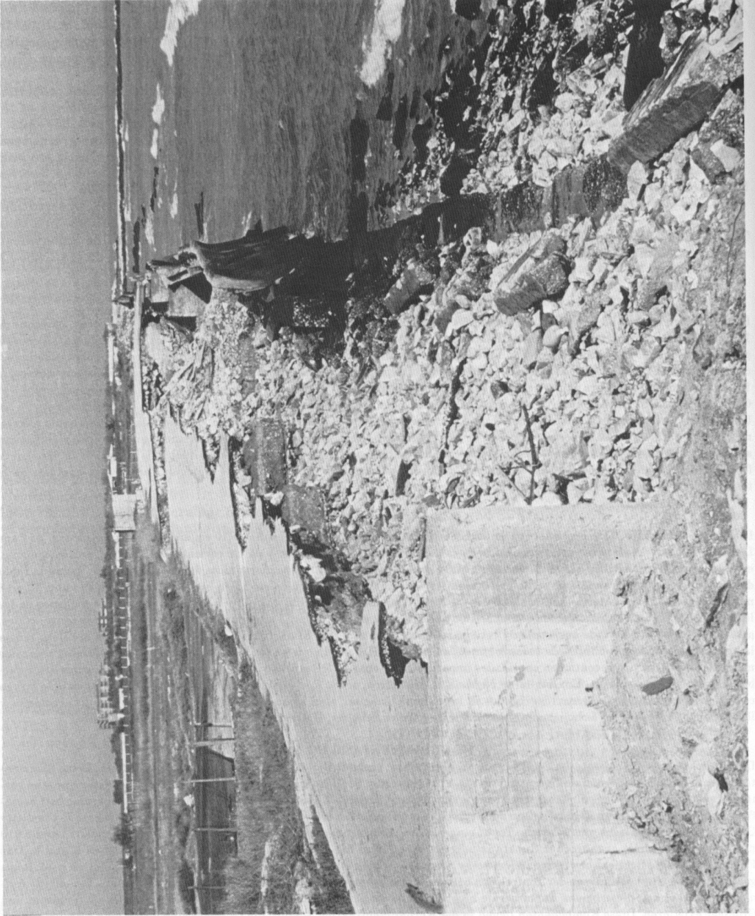
PHOTO 135. Destruction of seawall and highway along the Gulf of Manfredonia near Barletta, Italy. (Photo: H. Jesse Walker, Department of Geography and Anthropology, Louisiana State University, Baton Rouge, LA 70803).
