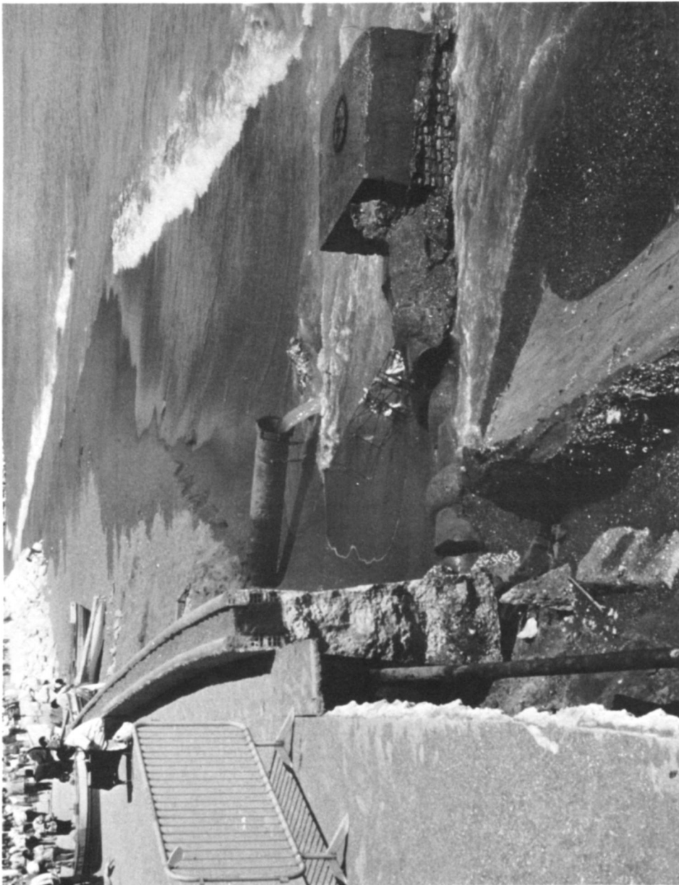
PHOTO 129. Beach erosion, caused by the interception of easterly moving longshore transport following the construction of a marina, has undermined the seawall at Torremolinos on the Costa del Sol in Southern Spain. This beach was over 50 m wide in 1970, but is now reduced to a few small, residual sand patches. The wall has fallen forward exposing the foundations, and fracturing the sewer pipe (centre of photograph) which is now discharging onto the beach. (Photo: R.W.G. Carter, Department of Environmental Sciences, University of Ulster, Coleraine BT51 1SA, Northern Ireland).
