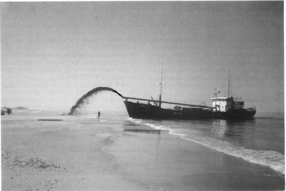
Figure 1(c). Dredge discharging over the bow, Danish North Coast (DANENA Dredging Co.).
