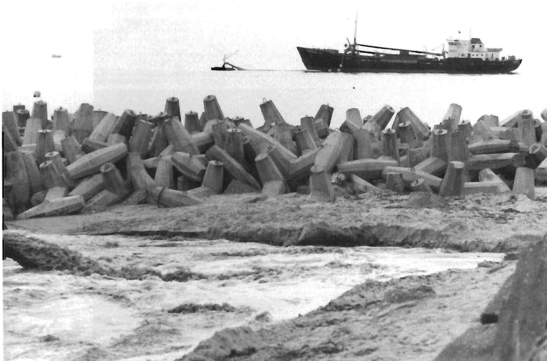
Figure 2(a). Hopper dredger with pump-out capability discharges material through offshore bottom terminal and permanent pipeline in the bottom. The Danish North Sea Coast. Coastal Directorate, 1985–1989.
