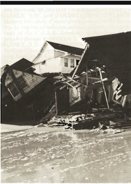
Figure 1. Storm damage along the Outer Banks of North Carolina.
