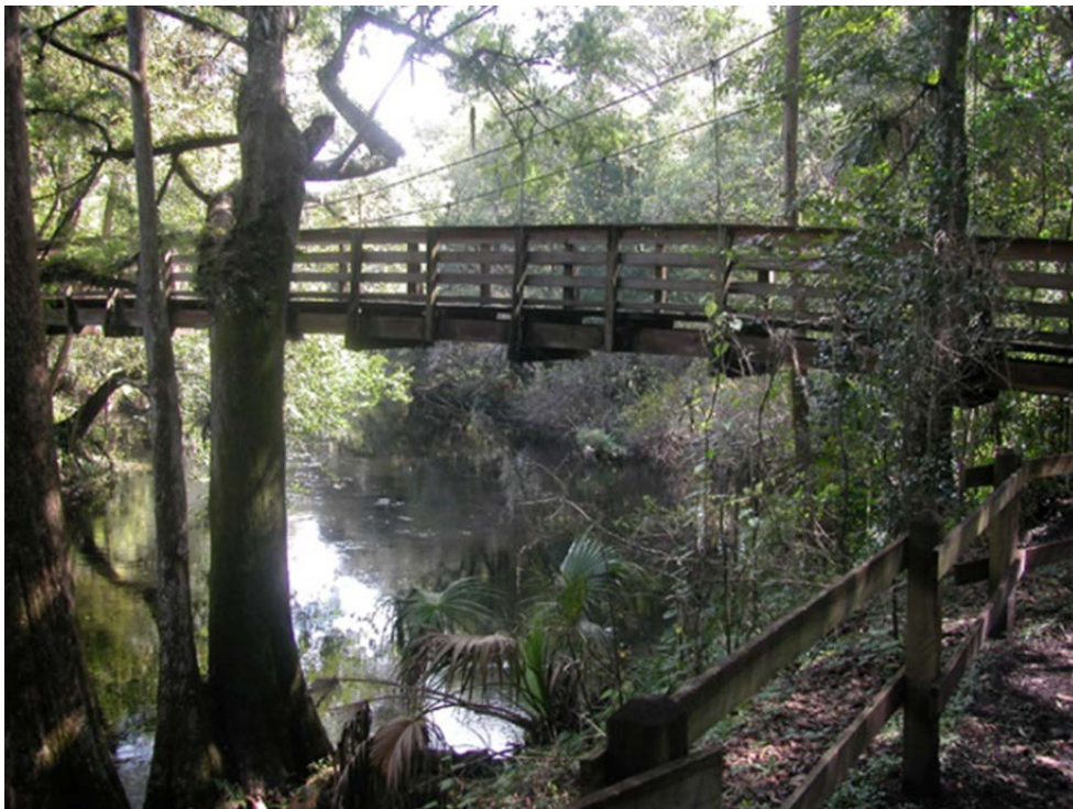
Figure 7: The CCC suspension bridge over the Hillsborough River in Hillsborough River State Park. Photo from Hillsborough River State Park web site ( http://www.floridastateparks.org/HILLSBOROUGHRIVER/DEFAULT.cfm ).
