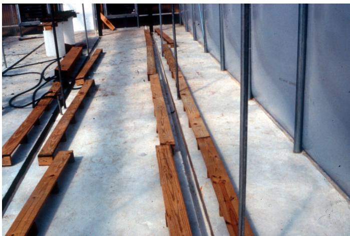
Figure 18. Drainage troughs created by pouring concrete floor around wooden forms and then removing forms, leaving behind troughs. Wooden benches also shown in photo.
