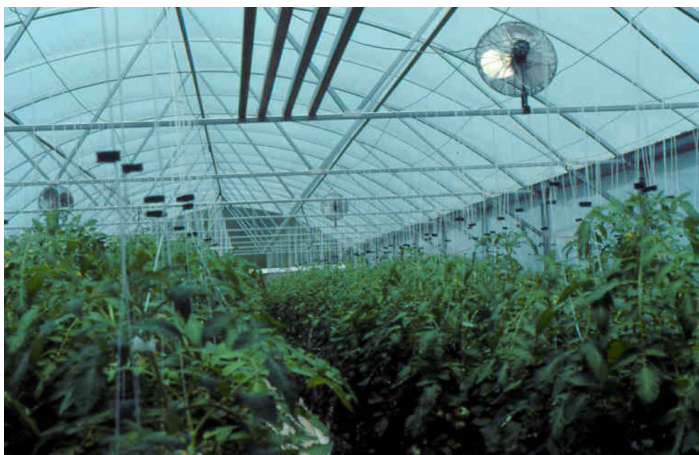
Figure 20. Horizontal air-flow fans.
