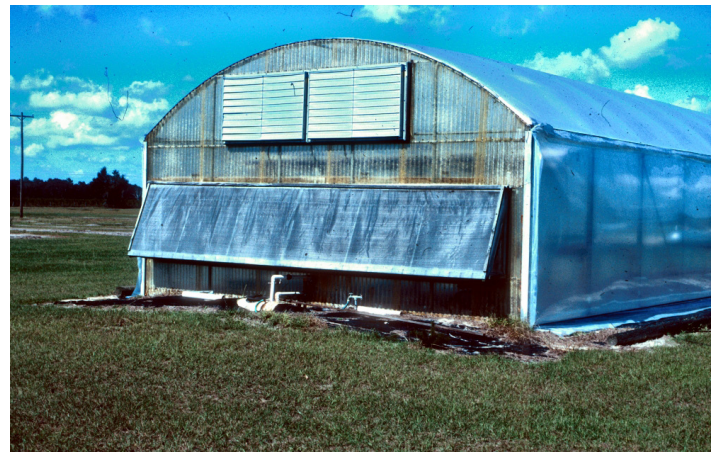
Figure 6. Cooling-pad endwall with open area for evaporative pad (in this photo, covered with motorized shutter) and 2 openings for motorized shutters, above cooling pad.
