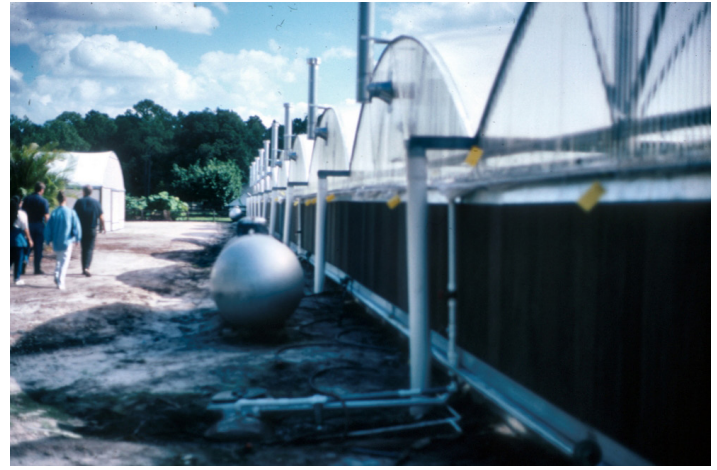
Figure 8. Evaporative cooling pad with underground water return system.
