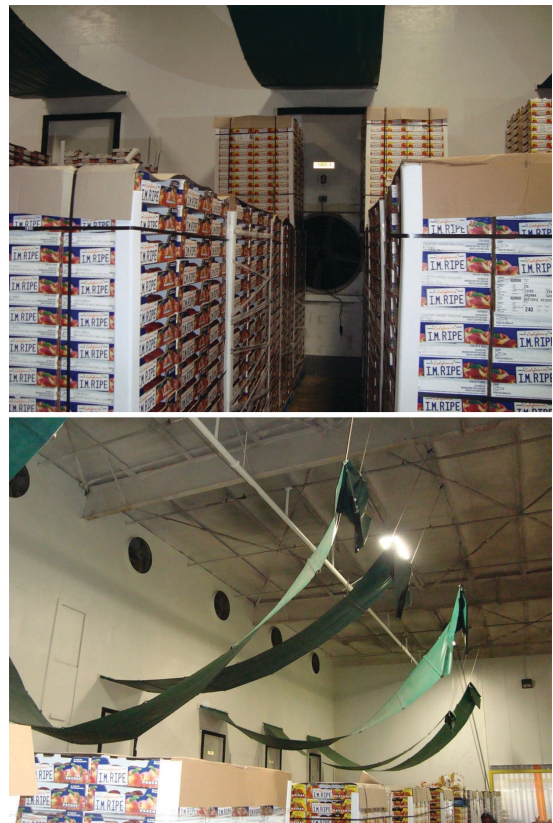
Figure 8-5. Forced-air cooling of peaches in palletized shipping cartons. The pallets have been aligned in rows on either side of fans set into the cold room wall to form the cooling tunnels, prior to lowering the tarps and turning on the fans to begin forced-air cooling. Credits: Jeffrey K. Brecht, UF/IFAS
