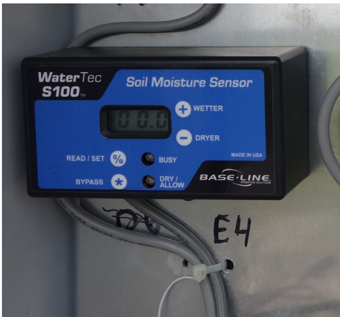
Figure 2. An example of a soil moisture sensor control panel. Credits: Michael Gutierrez, UF/IFAS
