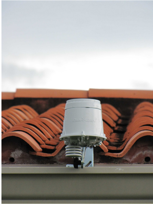
Figure 1. An example of an evapotranspiration sensor mounted on a roof. Credits: Michael Gutierrez, UF/IFAS
