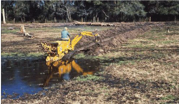
Figure 11. Digging drainage canals to remove standing water is one method to reduce mosquito larval developmental opportunities. Credits: CDC
