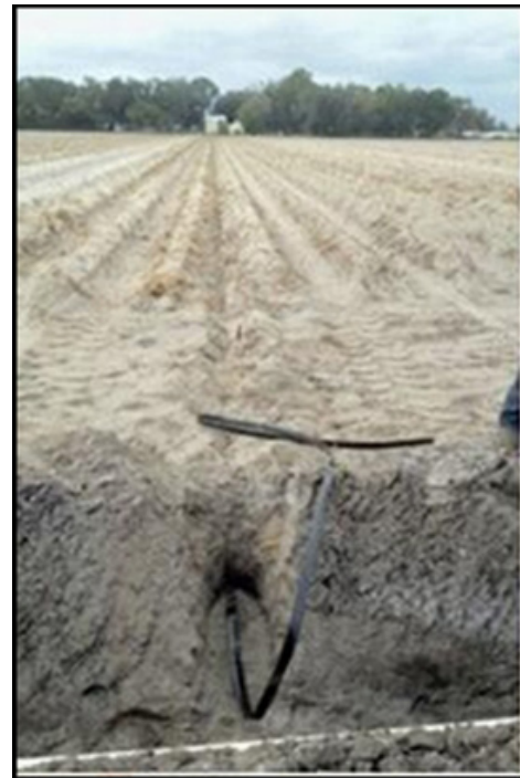
Figure 4. Installation of subsurface drip irrigation tape at a depth of 24 inches below the soil surface in a potato field in Hastings, Florida Credit: L. Zotarelli, UF/IFAS
