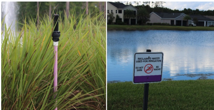
Figure 2. All reclaimed water piping, fixtures, valves, heads, etc. are required to be purple in color and labeled “Do not drink this water.” Credits: Terra Freeman, UF/IFAS
