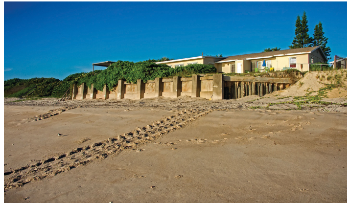
Figure 2. Example of a mixed wooden and concrete sea wall where a sea turtle was unable to nest. Credits: Gary Appelson
