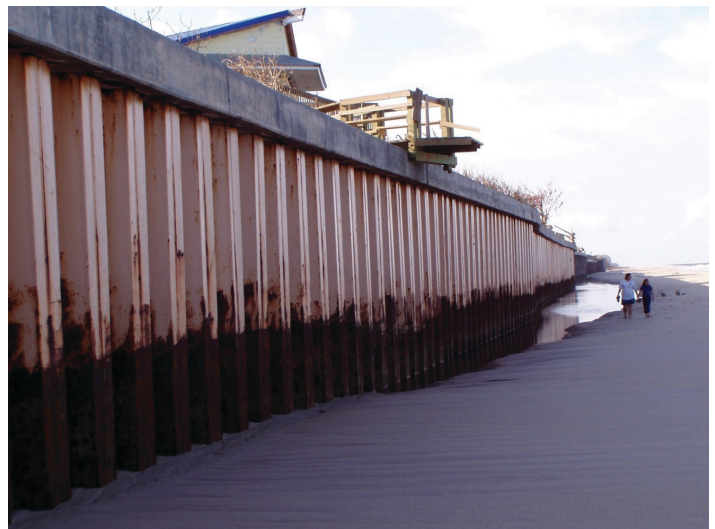
Figure 4. Example of a sheet pile wall where the beach dune system has been disrupted. Credits: Gary Appelson
