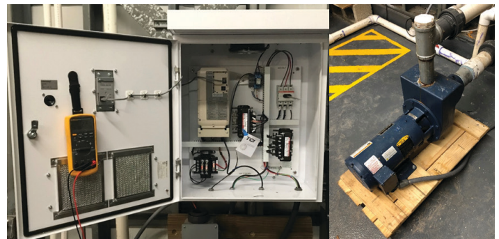
Figure 2. iQPump 1000 variable frequency drive (VFD) and control panel (left) used to operate the main water supply pump (right) at the UF/IFAS Tropical Aquaculture Laboratory. Credits: Jordan Neff, UF/IFAS
