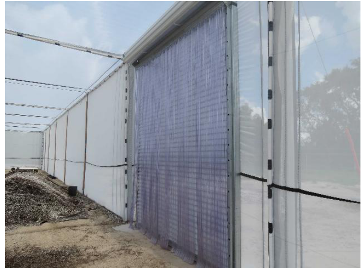
Figure 1. Steel roll-up door with a second plastic strip door, inside the UF/IFAS CREC CUPS. Credits: UF/IFAS
