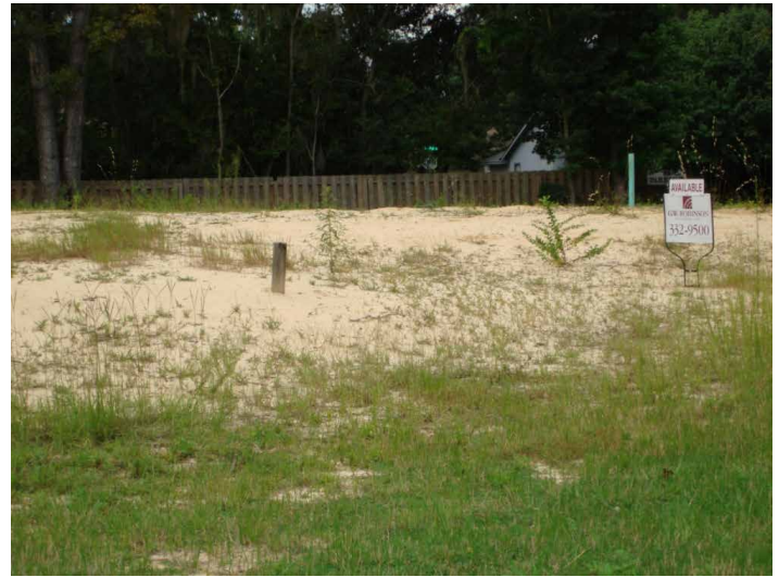
Figure 1. Fill sand is often piled on construction sites to serve as a base for the home's foundation. Credits: George Hochmuth
