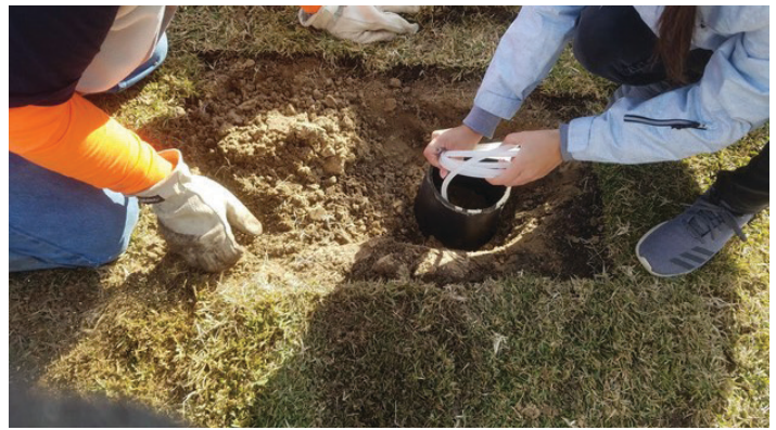
Figure 9. The soil profile is rebuilt, the access box is installed, and the collection tube is being rolled to be placed into the access box. Credits: Jovana Radovanovic, UF/IFAS
