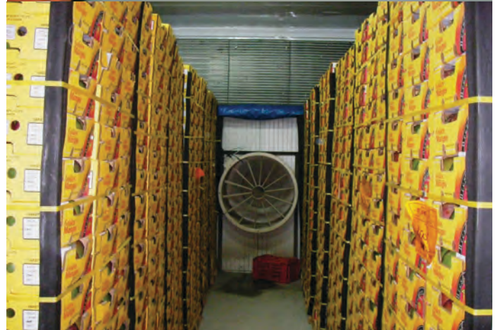
Forced-air cooling tunnels
