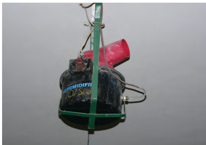
A storage room humidification unit
