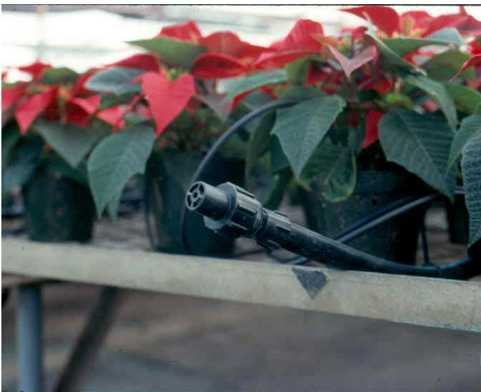
Figure 5. A low-pressure drain on the end of a pipe allows the pipe to drain rapidly when irrigation ceases. Credits: Tom Yeager
