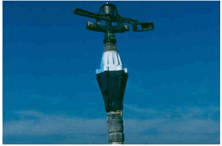
Figure 2. Appropriate nozzle operating pressure is achieved with a subtending regulator. Credits: Tom Yeager
