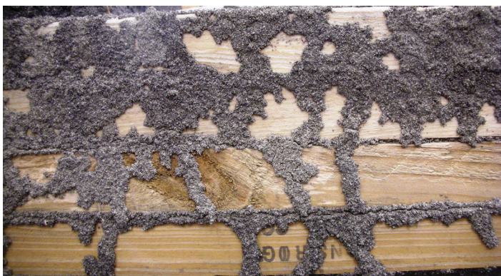
Figure 6. Subterranean termites use mud tubes to travel over exposed surfaces like hive supports. The “mud” is actually composed of soil, feces, and saliva. The tell-tale mud is the best indication of a subterranean termite infestation in your bee equipment or your home.
