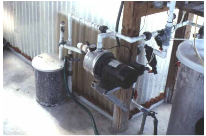
Figure 6. NFT recirculation pump and sump tank (note raised-neck opening to sump tank)
