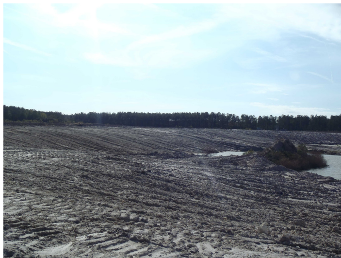
Figure 1. The future shores of a phosphate pit lake during reclamation to contemporary reclamation standards. Slopes on the lake exterior can be no steeper than 4H:1V (4 feet horizontal to 1 foot vertical) to at least 6 feet below the water's surface during seasonal lows. Credits: M. Wilson
