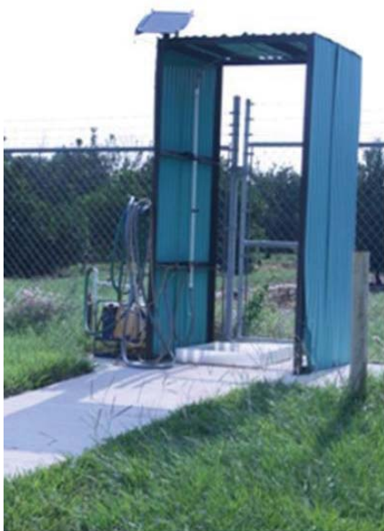
Figure 11a. Automatic personnel decontamination station
