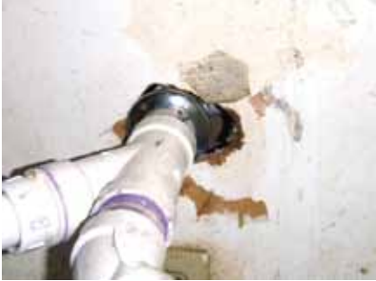
FIGURE 2 • An improperly installed escutcheon plate can be repaired by the college/university maintenance section.
