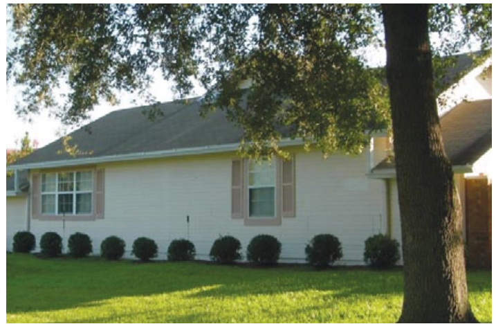
FIGURE 5. Shrubs along wall are overtrimmed.
