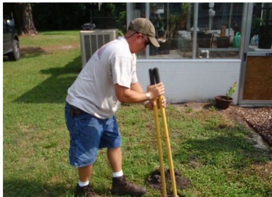
Figure 4. Dig a 2 ft hole. (Credit: B. M. Santos and T. P. Salame-Donoso)
