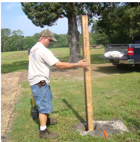
Figure 5. Hole for the supporting structure. (Credit: B. M. Santos and T. P. Salame-Donoso)
