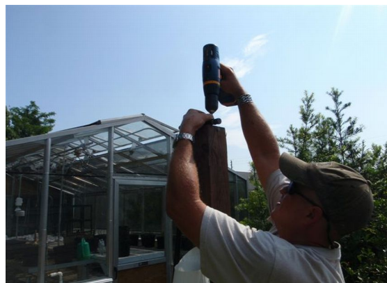
Figure 7. Install irrigation pipes on top of each pole. (Credit: B. M. Santos and T. P. Salame-Donoso)
