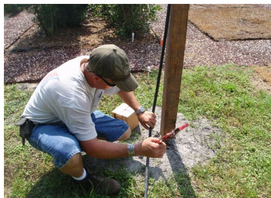
Figure 8. Set main pipe at the bottom of each pole. (Credit: B. M. Santos and T. P. Salame-Donoso)
