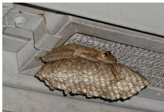
Figure 7. Cuban Treefrog perched on a wasp nest attached to a 12,470-volt substation circuit breaker. Fortunately, this frog did not cause a short-circuit. Credits: Kat Waters 2009
