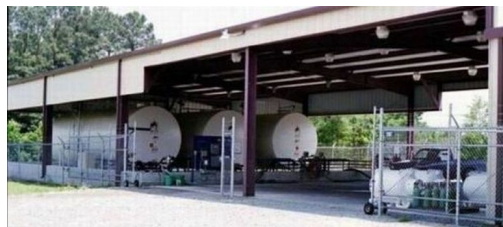
Figure 14. Large pesticide storage facility with bulk tanks within diking for containment and the area fenced for security.
