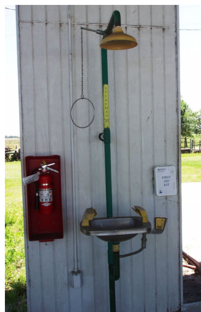
Figure 11. Permanent-plumbed decontamination site outside of a pesticide-storage facility.
