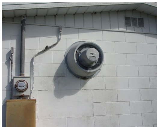
Figure 7. Exhaust fan at pesticide-storage facility helps reduce temperatures and remove dust and vapors from the facility.
