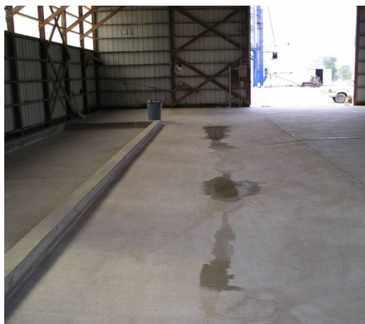
Figure 9. A recessed floor helps control spills or leaking pesticides.
