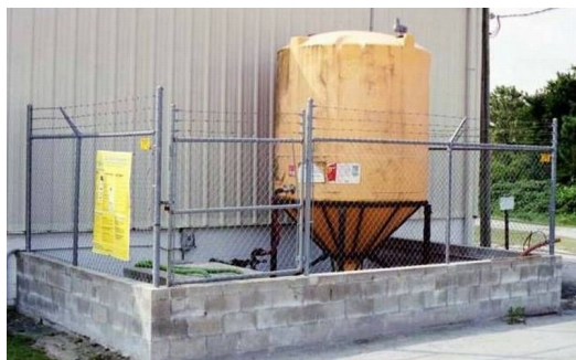
Figure 4. Pesticide bulk storage tank contained within a cinderblock dike.
