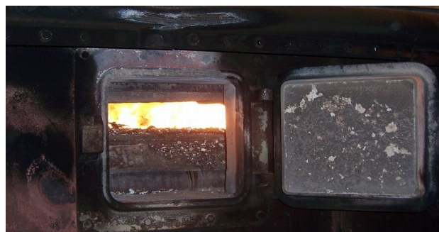
Figure 1. Wood can be burned in a boiler to heat water and generate steam. Credits: Lauren McDonell
