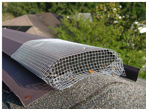
Figure 10. Preventative measures should be taken to discourage House Sparrows from nesting on urban structures. Here, hardware cloth is used to cover an open vent that might be an inviting nest site. Credits: Steve A. Johnson, University of Florida, 2008
