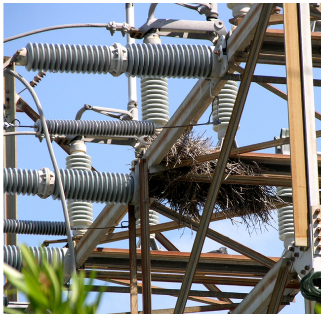
Figure 7. Monk Parakeets often nest on electrical utility structures, like this substation. When their nests become wet, they can cause short-circuit and power disruption, and are difficult and dangerous to remove. Credits: Steve A. Johnson, University of Florida, 2008
