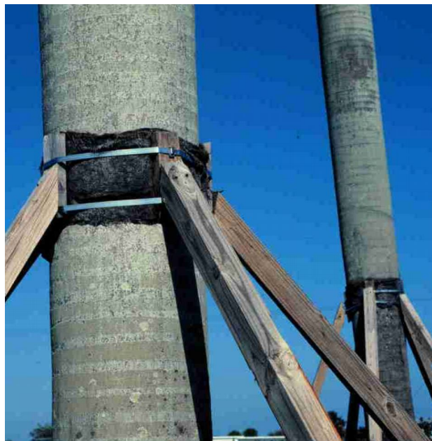
Figure 12. An excellent method of attaching support timbers to a palm trunk without damaging the trunk. Credits: Timothy K. Broschat
