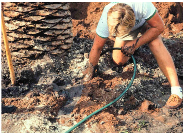
Figure 10. Using water to force sand under and around the rootball. Credits: Timothy K. Broschat
