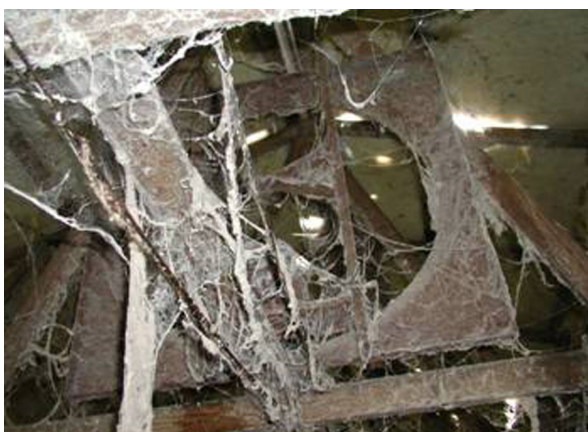
Figure 3. Broken fans and buildup of dust.
