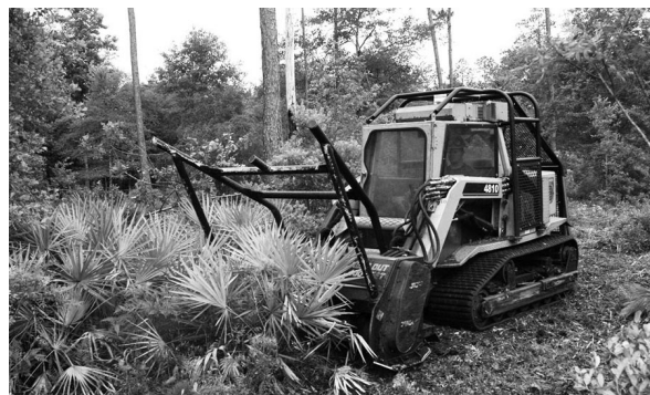
Figure 2. Machines like this Gyro-Track are used in interface neighborhoods to reduce understory vegetation. Credits: Larry Korhnak
