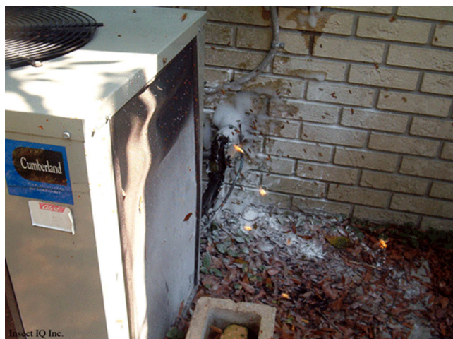
Figure 7. Honey bee colony that has become established in the wall behind an AC unit; foam has been used to eradicate the colony. Credits: AllFloridabeeeremoval. com
