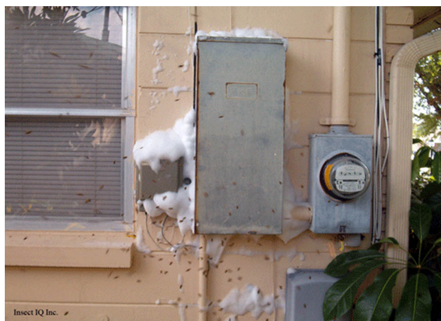
Figure 6. Honey bee colony inside power box; foam has been used to eradicate the colony. Credits: AllFloridaBeeRemoval.com
