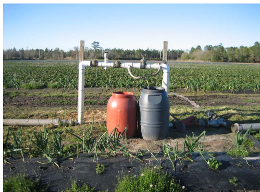
Figure 4. Back-flow prevention made of two ball valves and a vacuum breaker are placed upstream of the Venturi injector. Credits: Eric Simonne.
