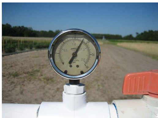
Figure 10. A fixed pressure gauge. Note the needle bathing in oil to prevent needle vibration and damage. Credits: Eric Simonne.
