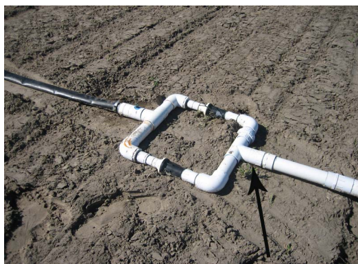
Figure 7. Pressure regulators are installed side-by-side in this system to allow a greater flow rate. Note the small injection port for chemical injection. Credits: Eric Simonne.
