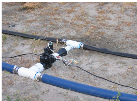
Figure 11. Solenoid valves connected to a timer allow sequential irrigation of different zones. Credits: Eric Simonne.
