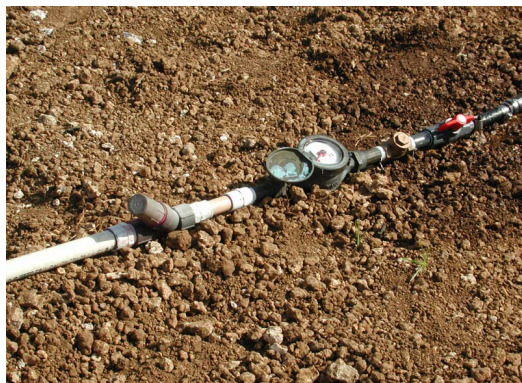
Figure 8. Water meters installed near the field. Credits: Eric Simonne.
