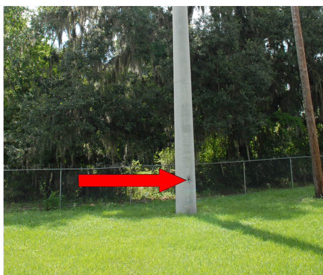
Figure 17. Small hole in light pole.
