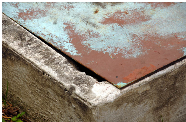
Figure 6. Crack in cement that creates opening.
