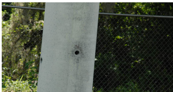
Figure 16. Small hole in light pole.
