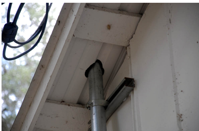
Figure 14. Opening around pipe.
