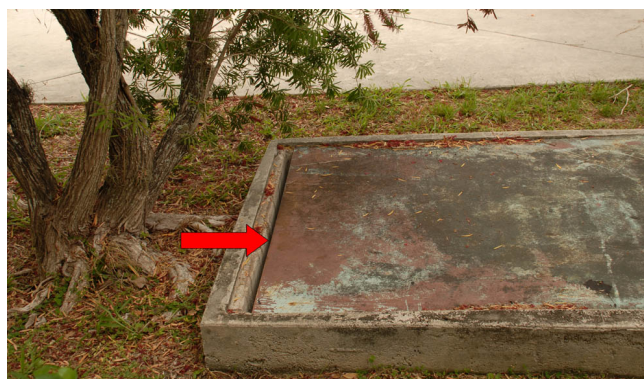
Figure 5. Open space in metal drain cover.
