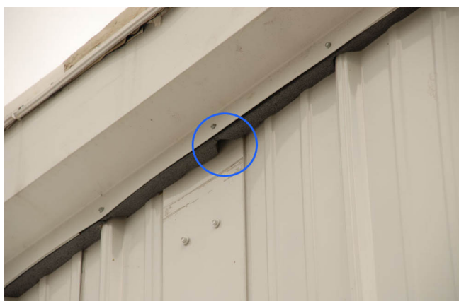
Figure 3. Small hole in siding.
