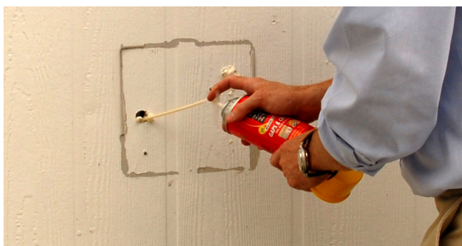
Figure 21. Foaming holes in side of building.
