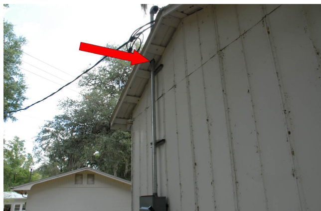
Figure 13. Opening around pipe.
