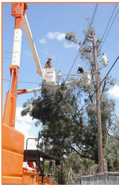
Figure 3. Working near power lines is an especially dangerous situation.
