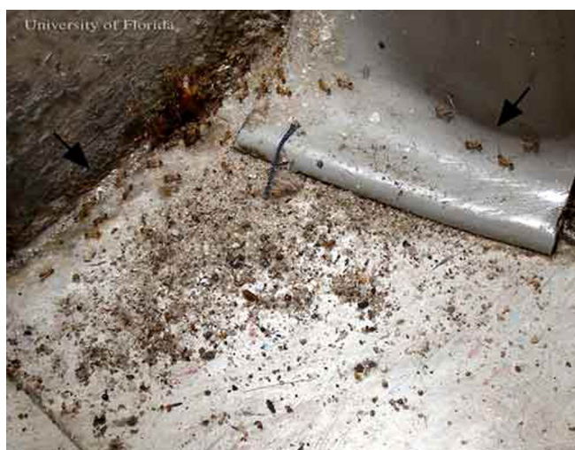
Figure 2. Debris caused by bigheaded ants, Pheidole megacephala (Fabricius), inside a structure on a tiled floor. Arrows indicate trailing ants. Credits: R.H. Scheffrahn, University of Florida
