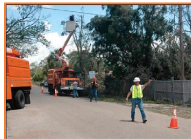
Figure 3. Appoint a flagger or use barricades and warning signs to control traffic or onlookers.
